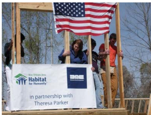
Above: Students help build a house on Ferry Street in New Orleans
